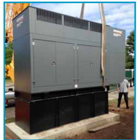
The Rushford at Meriden generator project has been completed. Workers are shown lowering the generator into place near the building's administrative entrance last Friday.
